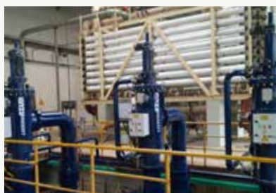
3x AZUD LUXON LDB 13200 S/14 Shandong water reclaim
