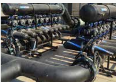
2x AZUD HELIX AUTOMATIC 4DCL9 AGBAR Santiago WWTP
