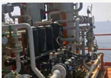
AZUD HELIX AUTOMATIC 703 SW AA ENI Ancona oil platform
