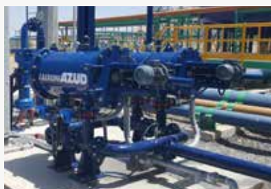
2x AZUD LUXON LXE 2700 S/4 OCP Khouribga phosphate mine
