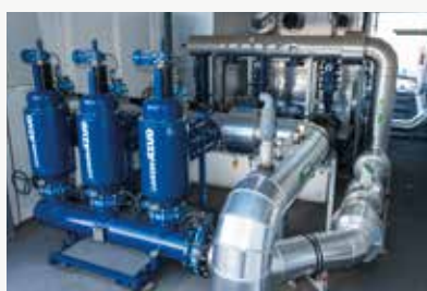
3x AZUD LUXON LDB 5400 S/8 Mould injection machine circuit
